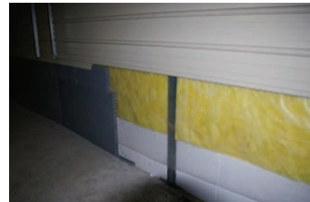
Picture: Efficient wall structure where the lowest part of the wall is planked with PVC boards inside and lowest an insulation with polystyrene and further up—fibre glass. Further up the inside wall is in steel
