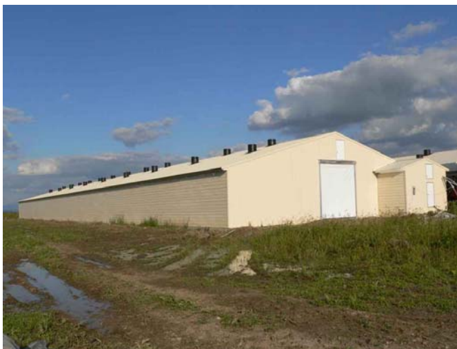
Picture: 2 chicken houses in Odoreu, Romania (100 x 20 metres) - ready to produce high quality broilers.
